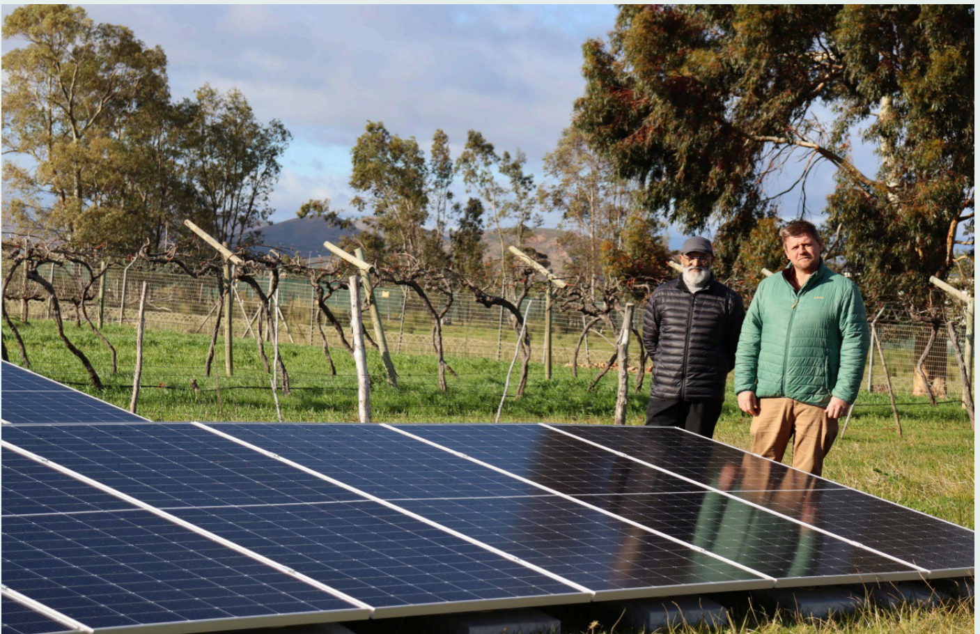
Mr Vincent Uys (Senior Educational Specialist in Agriculture: Farming Management & Entrepreneurship) and Mr Derrick Matthee (Acting Campus Manager: Worcester Campus) at the newly installed solar panels on campus
