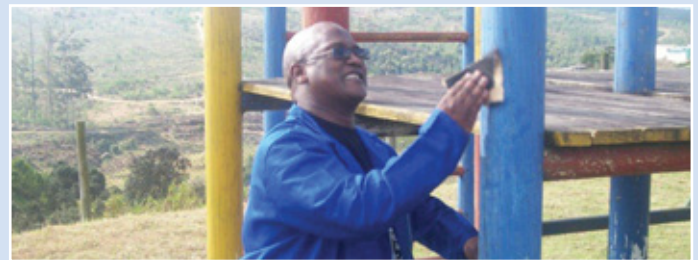
CEO painting: proving that CEO skills can be utilised for more than strategic meetings, Mr Luvuyo Ngubelanga sanding some jungle gym equipment to ready it for a new layer of paint
